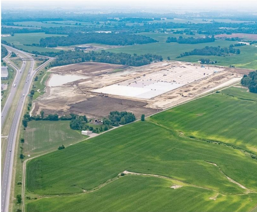
In May, Philadelphia-based discount retailer Five Below broke ground on its planned $100 million Midwest distribution and e-commerce center, the county's first distribution center.
